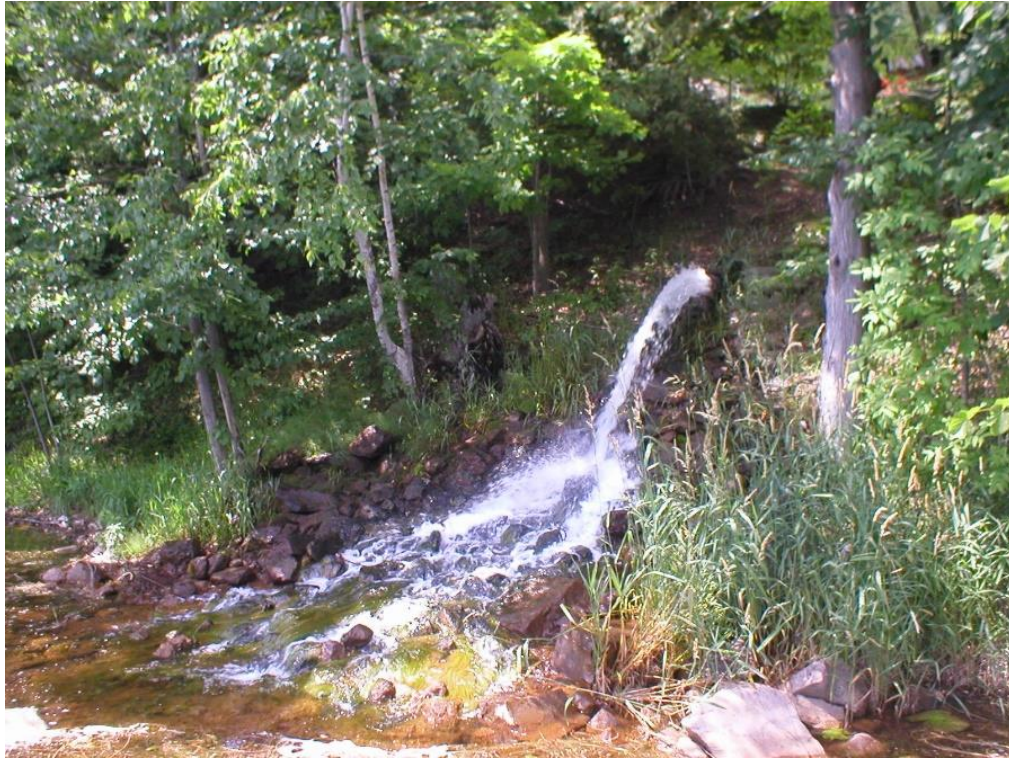
500 gallon per minute well installed in 1972
